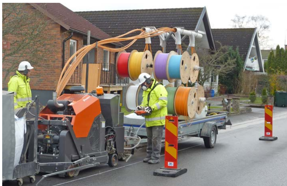
The first step is to saw a trench through the surface of asphalt or concrete into the underlying bearing layer. At the same time a number of ducts for fibre cables are put in the bottom of the trench.
